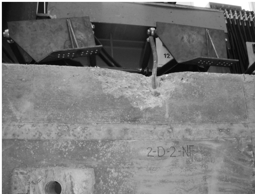
Figure 1: Concrete Delamination Failure
